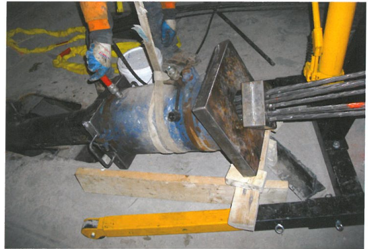
Tensioning jack on top of gate applying 250,000 lbs. of tension to the new grouted DCP post-tensioned trunnion anchors which are located about 8 ft. below.
